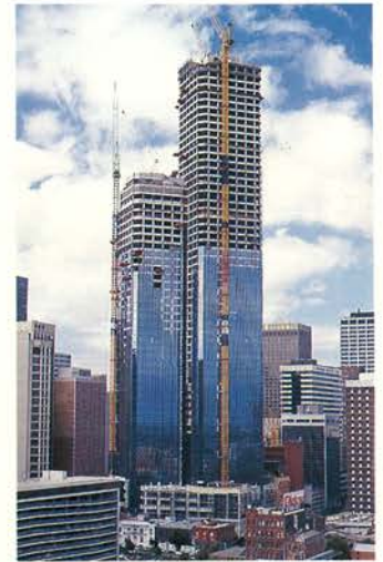
In Melbourne the Rialto Building, shown here half-finished in 1984, became, at 242 metres, the tallest building in Australia when completed in 1985. Its 56 levels included an international hotel, 86 thousand square metres of office space, a 260-seat conference auditorium and parking for 650 cars. Australian property, 1985.
